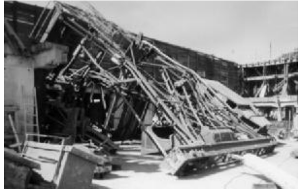
The gantry of the coal discharge plant at Blackwattle Bay after it was "dismantled"
