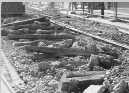
Sleepers revealed during the Glebe Point Road upgrade. Photo: Jan Wilson, 13 October
