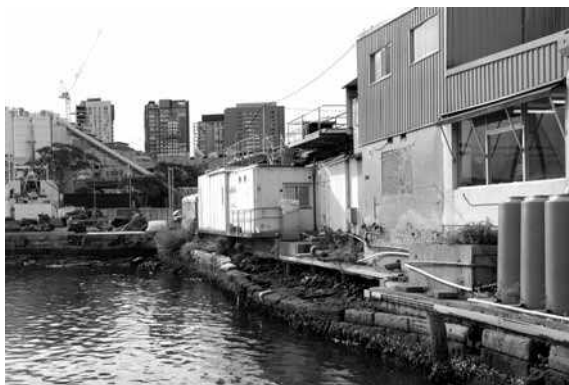
The decaying sea wall behind Claudios will be repaired and incorporated into a bayside park.
