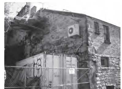
The ruins of Sydney Leadworks today. Photo: Rod Holtham
