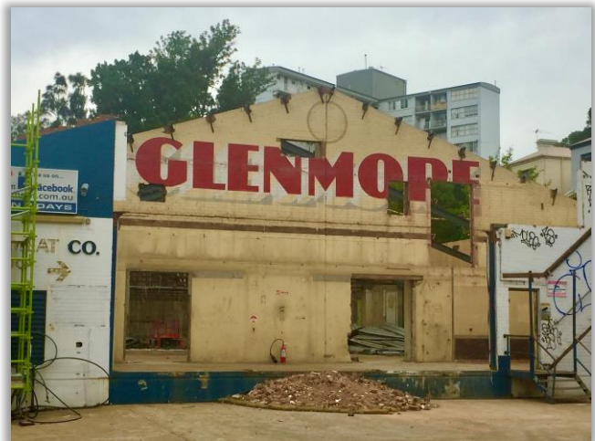
The site as it was in February 2020; the Glenmore Meats building is partly demolished (photo: Phil Vergison)
