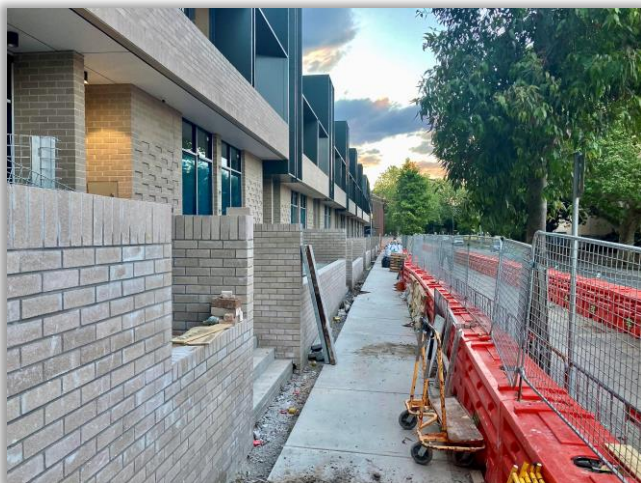
The apartments that are nearing completion on the former Glenmore Meats site (photo: Phil Vergison)
